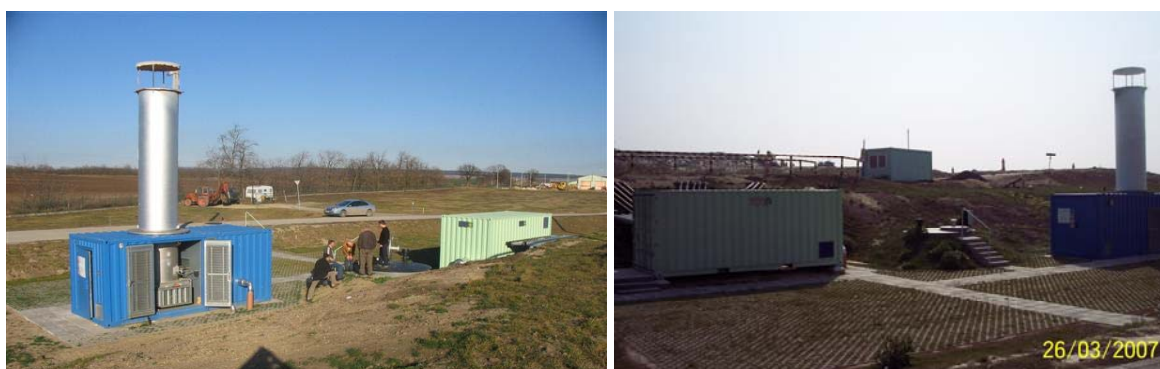
Figure 10: booster & flare, condensate shaft and manifold station in spring time 2007
