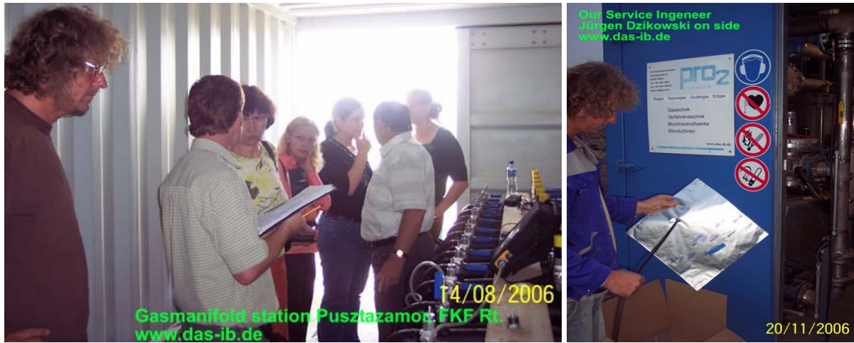
Figure 9: Measurements and optimisations during the test phase of degasification
